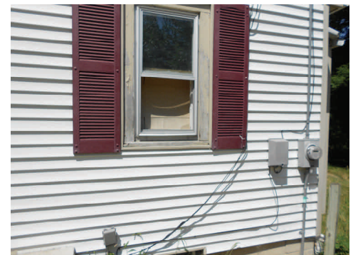
Broken windows and wires out of place
