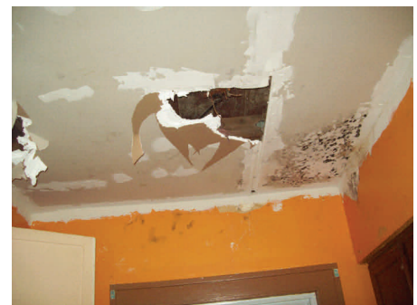
A leaky roof allowed water into the house damaging the ceiling and prompting mildew to develop.
