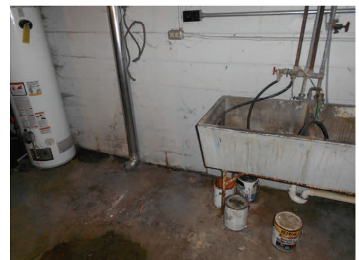
A leaky basement with lots of potential
