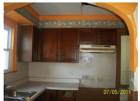
Kitchen cabinets were missing doors and drawers. The stove hood was grimy, and no appliances remained in the house.
