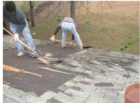
Workers remove shingles and prepare to repair holes in the existing roof. A complete new roof was installed.
