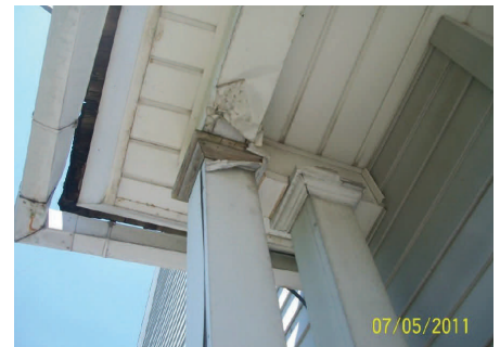
The wrap is coming undone and wood rot was found on the roof decking. Wrap arounds for some windows were also a problem.
