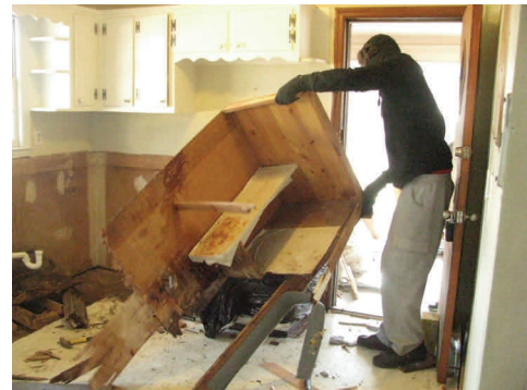
Old cabinets, which were in disrepair, were removed, and the entire kitchen was gutted for a full rehabilitation, including energy-efficient appliances.
